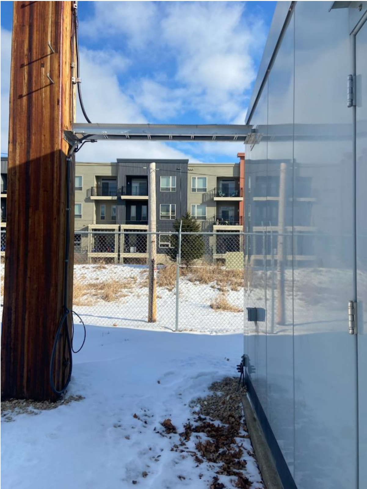
Similar facilities installed by MGE
